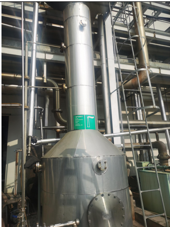
甜菊糖浓缩冷凝废气排气筒 DA008
